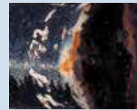
Without zinc protection Corrosion beyond notch
