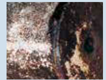
With zinc protection Zinc salts on notch
